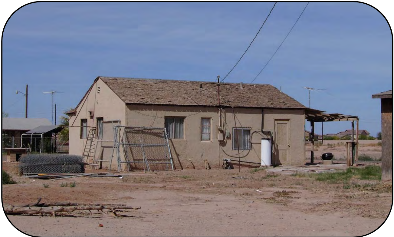
Figure 12: Old Town Housing with Code Violations
