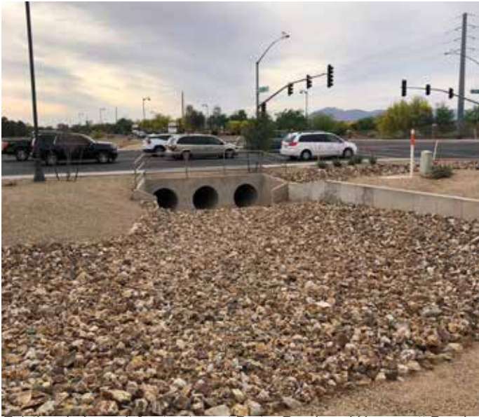
Existing drainage infrastructure at Porter Road and Honeycutt Road
